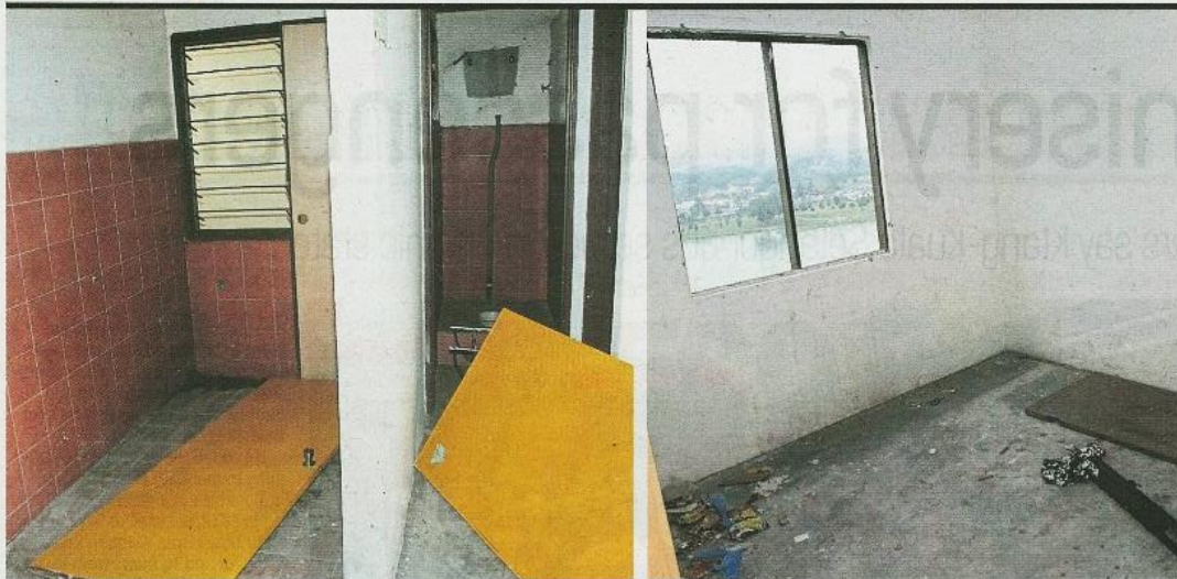
Deserted: Empty units with broken doors and missing windows in PPR Cempaka in Pantai Dalam (left) and PPR Intan Baiduri (right). Some quarters think that DBKL should fix it up and give it to the hardcore poor.
