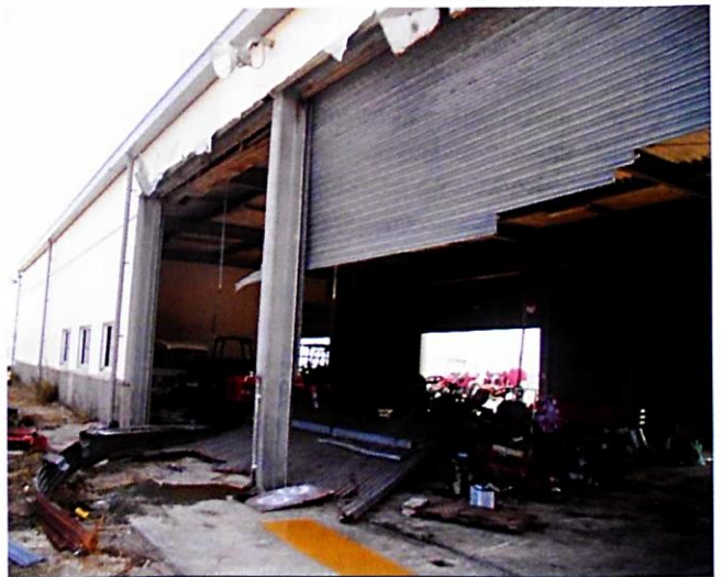
Photo 3 Example of damage caused by typhoon (Miyakojima, Okinawa in 2003)
