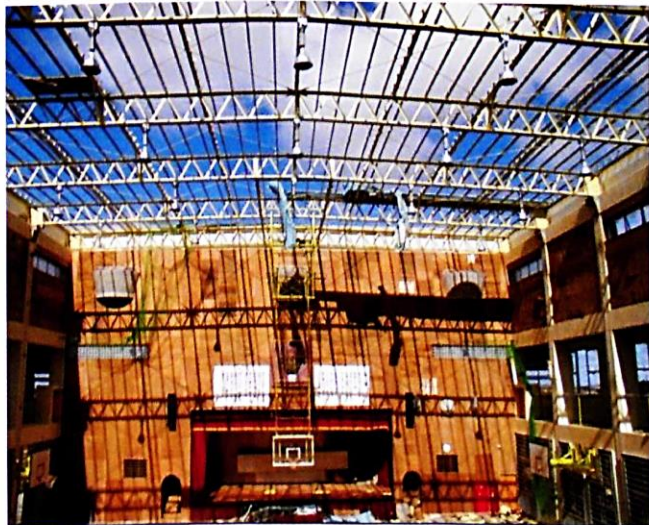
Photo 2 Example of damage caused by typhoon (Miyakojima, Okinawa in 2003)
